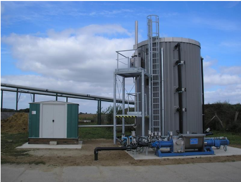
Fig. 2: Pilot plant (recent type) of High-Performance-Digester at pig farm
