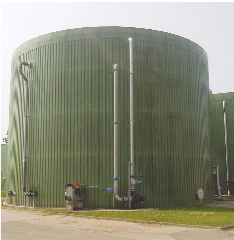
Fig. 3: Biogas plant (standard type) of High-Performance-Digester at cattle farm
