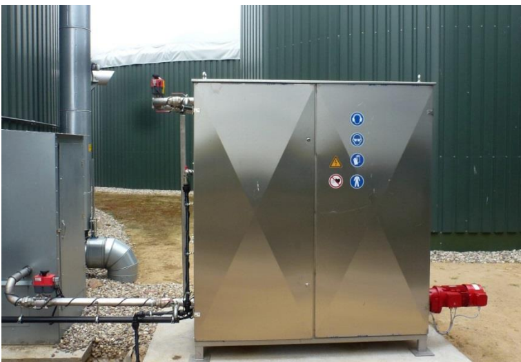
Fig. 3: Wave-Box installation with Kombi-Hydrolysis
